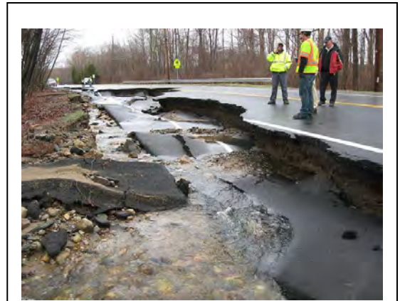
Road damage in Hopkinton from the 2010 floods. (Photo Credit: RI DOT)
