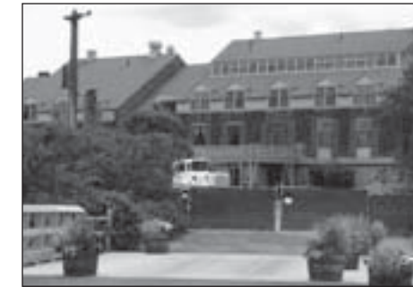
Construction fencing and drill rigs define the look of the Weekapaug Inn this summer
